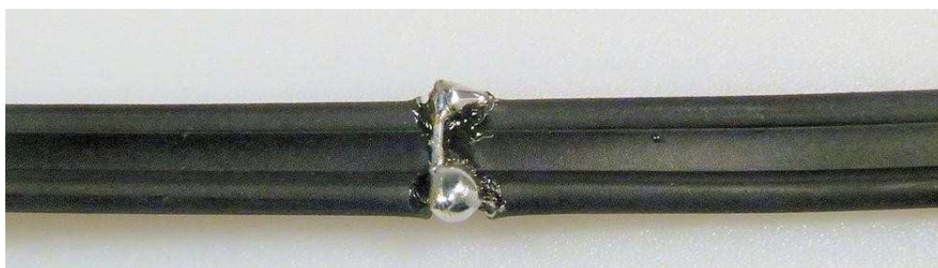
Photo 4.2.4. Short circuit location
