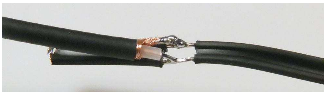
Photo 4.2.5. Connection of power supply cable
