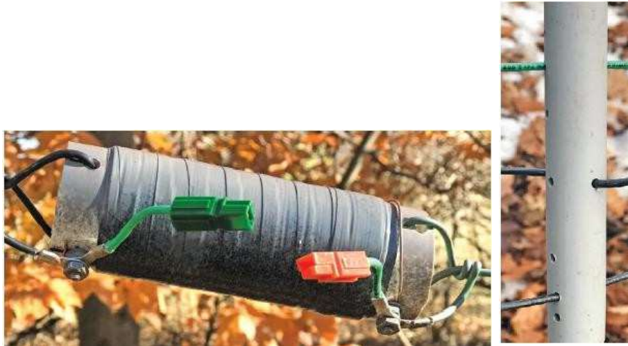
Photo 1.1.5.5. Extension coil for 80 m band without connected jumper. The coil is wrapped with insulating tape to stabilise the winding and protect it from environmental influences. The coil has been painted grey for aesthetic reasons. On the right is the wire for the 80 m band and on the left is the main part of the dipole for the 40 m band
