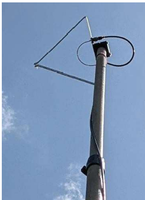
Photo 4.3.3. Antenna mounted on mast
